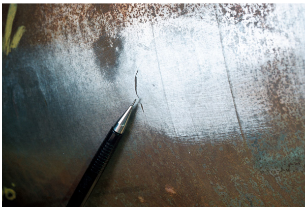
Fig. 11 Close-up of one of crack locations identified in Fig. 10
