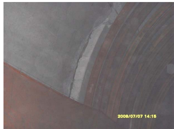
Figure 10 Lining structure damage observed in the Longxi tunnel
