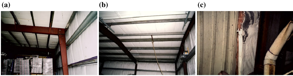
Figure 6. Metal building insulation applied to the walls and ceiling of the facility (a) Component L (b) Component N (c) Component D.
