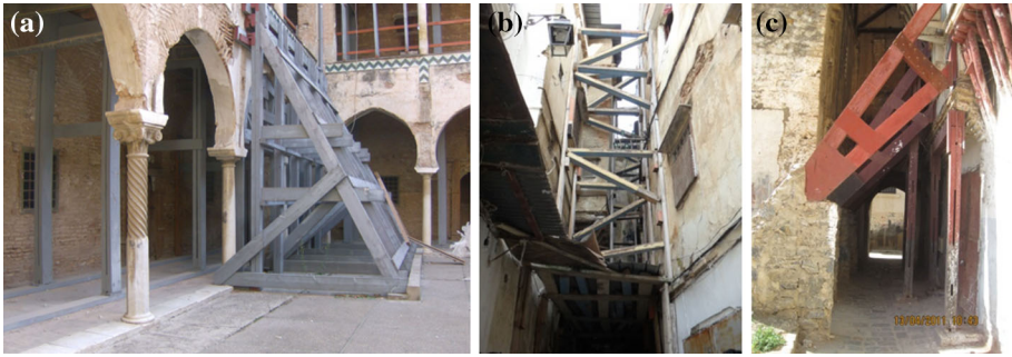
Fig. 17 a Shoring system made of wooden trusses used to prevent out of plane failure of masonry walls in The Casbah of Algiers, b shoring system applied to buildings facing a narrow street and c system of shoring also supporting the q'bu
