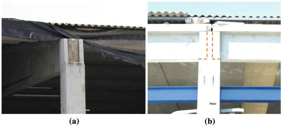
Fig. 7 a Seating of double slope precast beams showing the fork at the top of the column : seating at an end column . b Seating at an intermediate column of a “T” section beam (with dashed lines indicating the section of the beam at the seat pocket)
