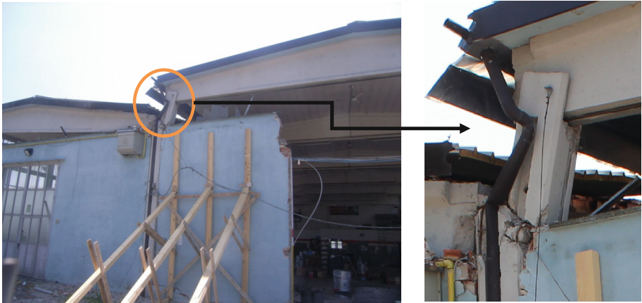
Fig. 10 Loss of the left girder seating due to the interaction with masonry panels (short columns/shear failure)
