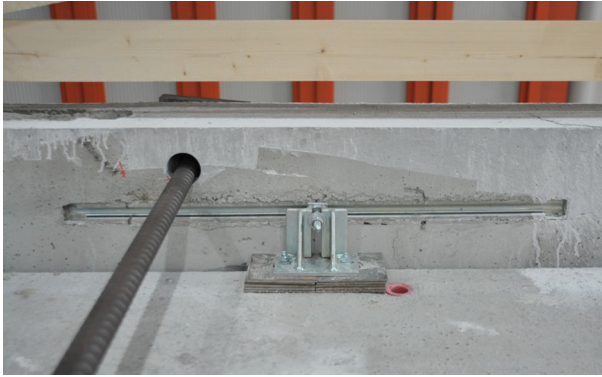
Fig. 22 Panel connection device that provides resistance in the vertical and out-of-plane directions and accommodates large relative deformations in the lateral direction
