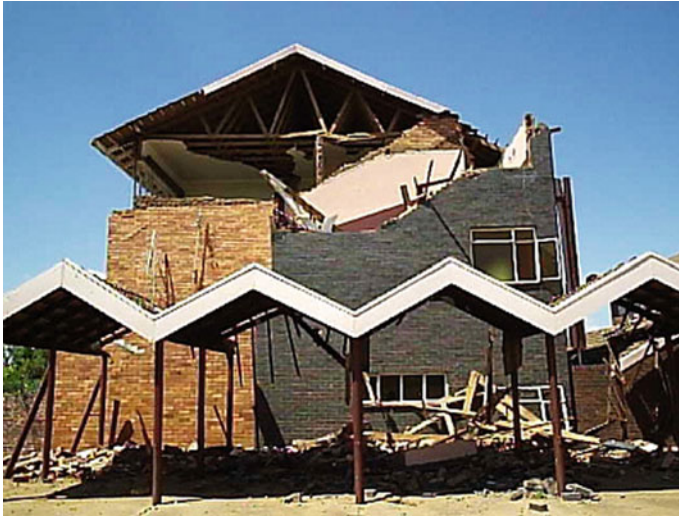
Fig. 1 Damage to brick masonry wall caused by M_L 5.3 rockburst from March 9, 2005 in Stilfontein, South Africa (courtesy of A. Cichowicz)
