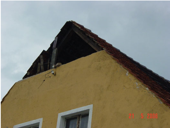
Fig. 2 Damage to a gable wall caused by M_L 4.3 rockburst from May 21, 2006 in Polkowice, Poland (approximately 600 m from epicenter)
