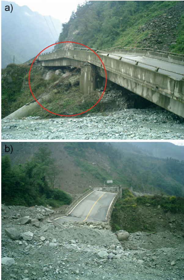
Fig. 11 Structural damage to the highway between Chengdu and Yingxiu. a View towards Chengdu. A collapsed column is visible in the lower left corner. b View towards Yingxiu, where the road section in the foreground is dislocated and separated from the section in the background
