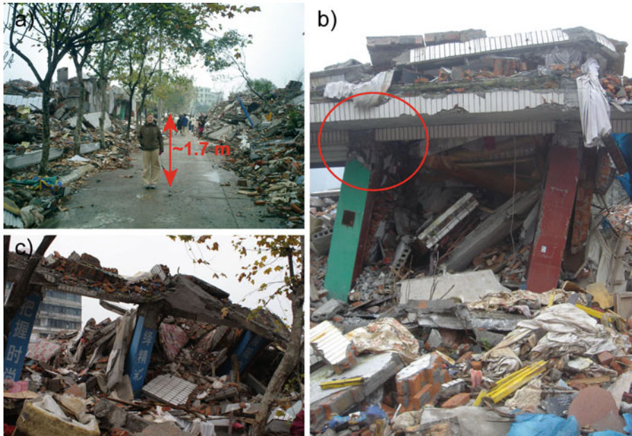
Fig. 8 Typical market buildings with shops on the ground floor and apartments on the second floor, Hanwang. a View through the main street of the market area. b Close-up of the structural damage of the beam-column joints in a market building. c Front of market building is partial collapsed while the rest of the building is totally destroyed
