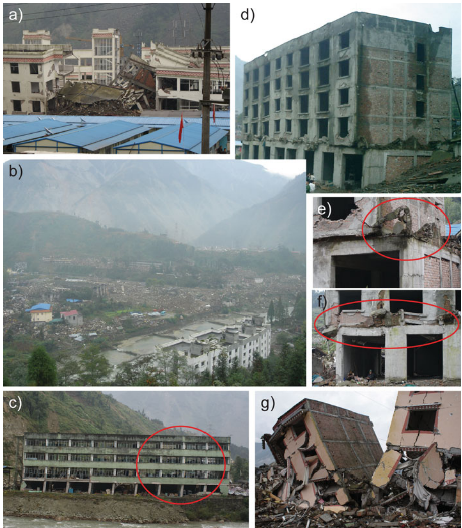
Fig. 4 Building damage at Yingxiu Town of Wenchuan County. a Xuankou Middle School, shelter buildings are visible in the foreground. b Overview of Yingxiu where ca. 80% of the city's buildings collapsed during the earthquake. c Factory building with clearly tilted columns. d–f Six-story RC-brick infill building which suffered a single story collapse of the second floor. g Partial collapse of residential buildings
