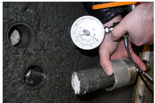
Fig. 16 Adopted procedure for in situ measurements of tensile bonding strength. Top conceptual diagram showing the layout of the test. Middle Preparation with over-coring with grinding of the test specimen. Bottom in situ specimen after testing
