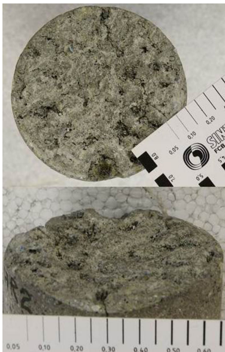
Fig. 8 Example of recordings of cracks in a sprayed concrete surface using a concrete crack measurement gauge
