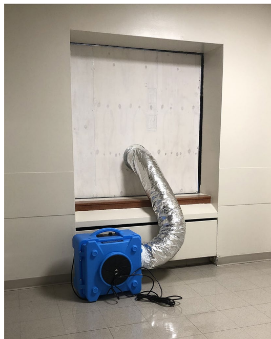
Fig. 1 Telemetry room converted to a negative pressure environment using an extractor fan with HEPA filter to a board covering an exterior window to create a temporary ICU room
