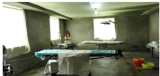
Fig. 4 Operation room, in which two operations can be carried out at the same time
