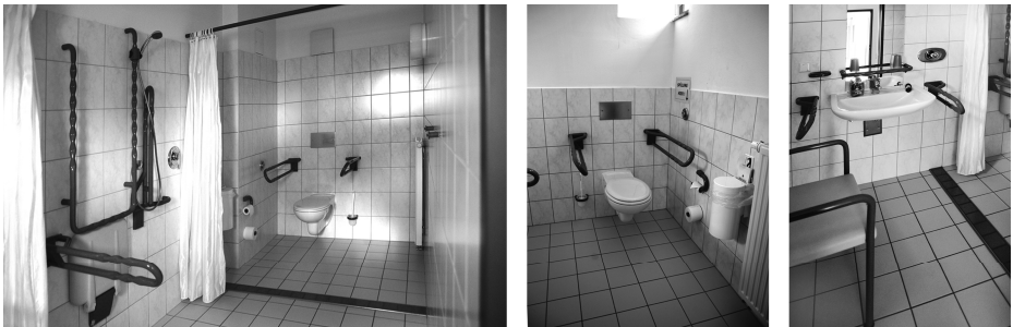
Fig. 4. Windmühle Seifhennersdorf – adjusted bathrooms for disabled users (from the left – in a large hotel, in a restaurant, details of a sink/basin installation)
