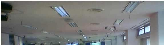
Fig. 4. Ceiling of the South Laboratory with installed sensors
