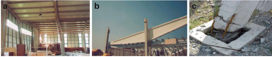
Fig. 8.2 Observed damages. (a) Out of plane deformations of plane frames; (b) Collapse of a rigid roof beam; (c) Plastic hinge at column base
