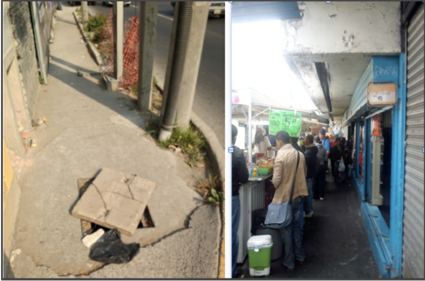
Fig. 2. Infrastructure and sidewalks problems
